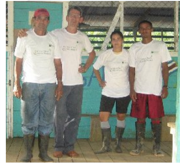
The our partner team performing repairs at a local school in Costa Rica
